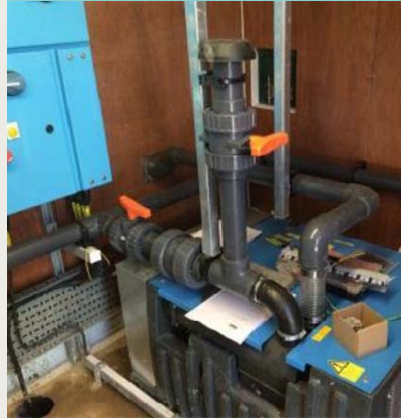
View of vacuum pump inside siphon control kiosk located at the siphon crest.
