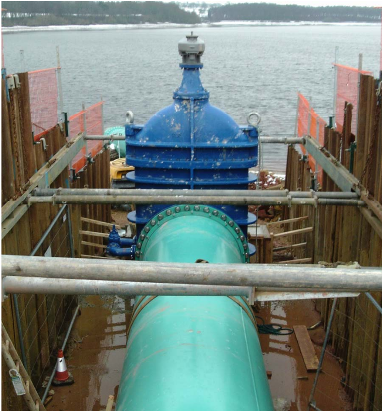
View of Gate Valve installed at upstream edge of dam crest.
