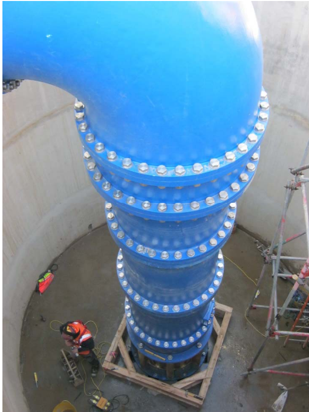
View of Submerged Discharge Valve in circular chamber.
