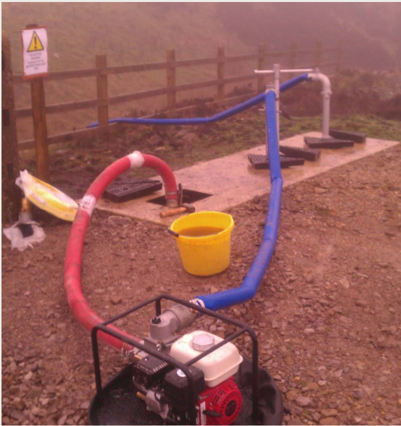
View of the pumped priming arrangement during commissioning.
