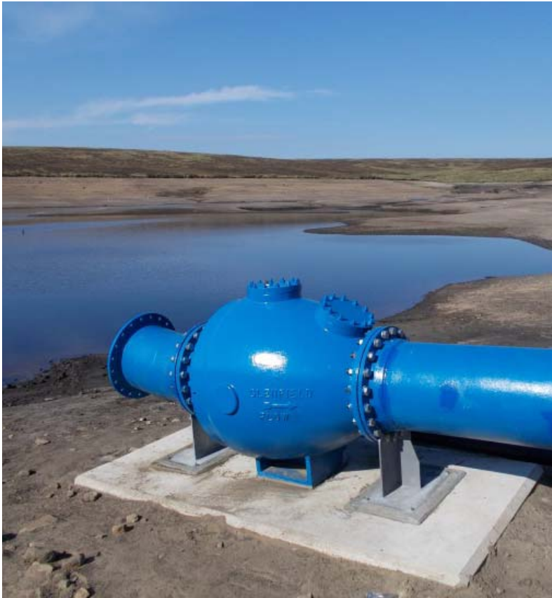
View of the non-return valve at inlet of siphon pipe during construction.
