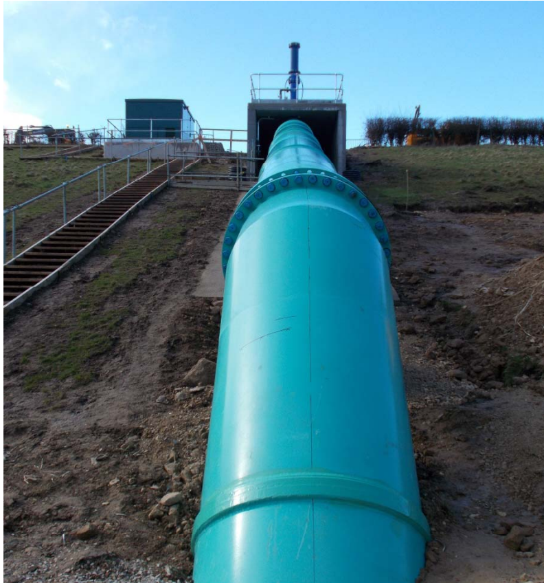
View of downstream leg of siphon pipe, looking towards the crest and siphon control kiosk.
