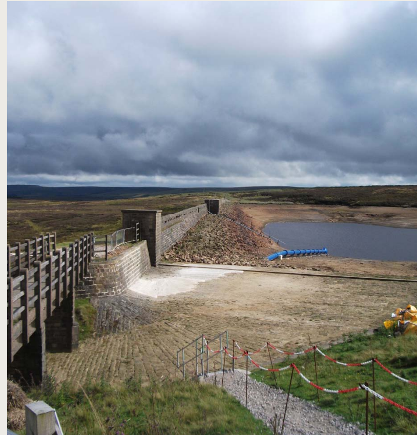
View of Keighley Moor Reservoir near the end of the construction phase.
