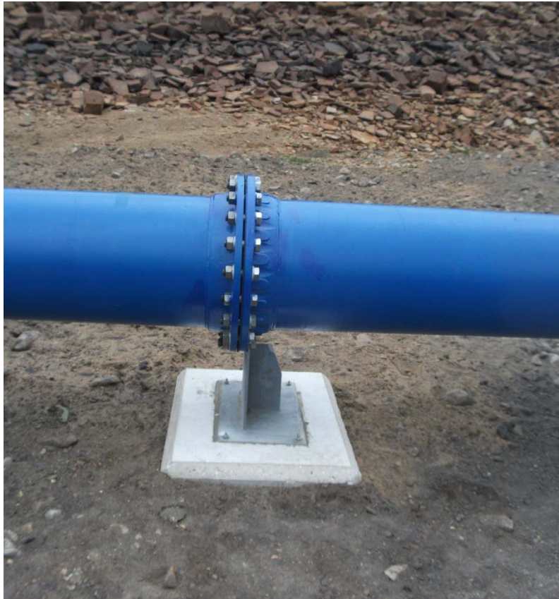
View of pipe supports on upstream leg of siphon.
